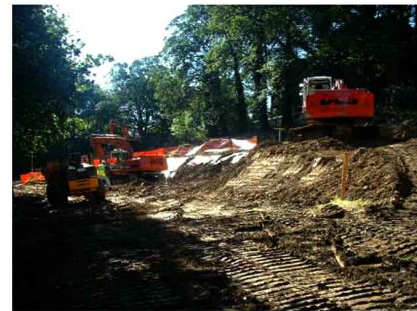
An unprotected site with excavations causing severe harm
